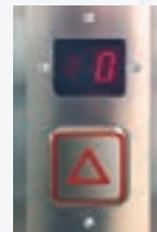
Door operating panel with floors light indicator
